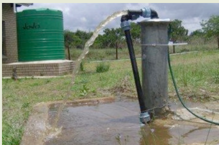
The new electric pump in action.
